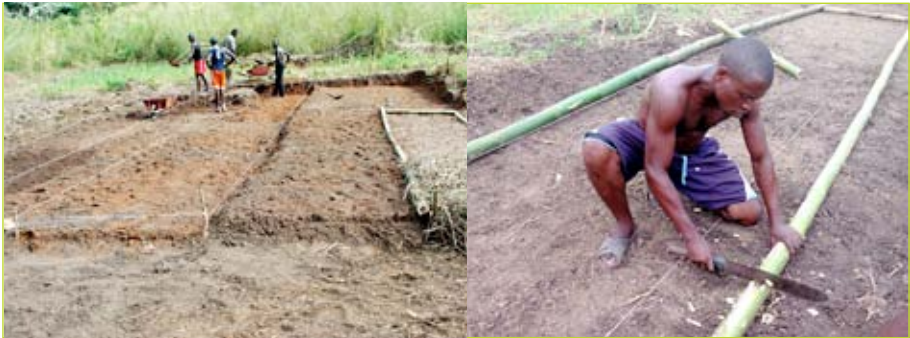
Marking of the compartments and cutting of 14 m and 1.5 m long bamboos sections for the installation of 4 adjacent 1000 acacia compartment, J. Scholle, GRET, DRC, 2014.
