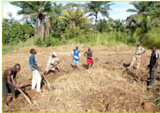
Leveling the location after marking the nursery's perimeter, J. Scholle, GRET, DRC, 2014.
